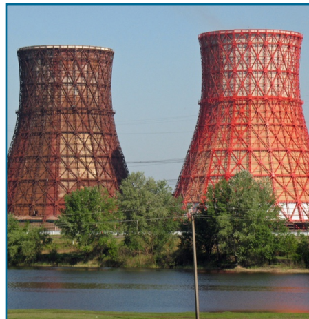
Figure 5. Hyperbolic Cooling Towers (Source: Victor Vizuz).
